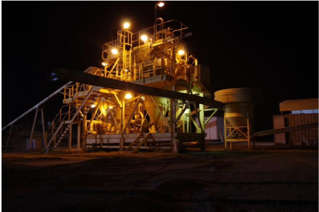
The processing plant has the capacity to work at night
